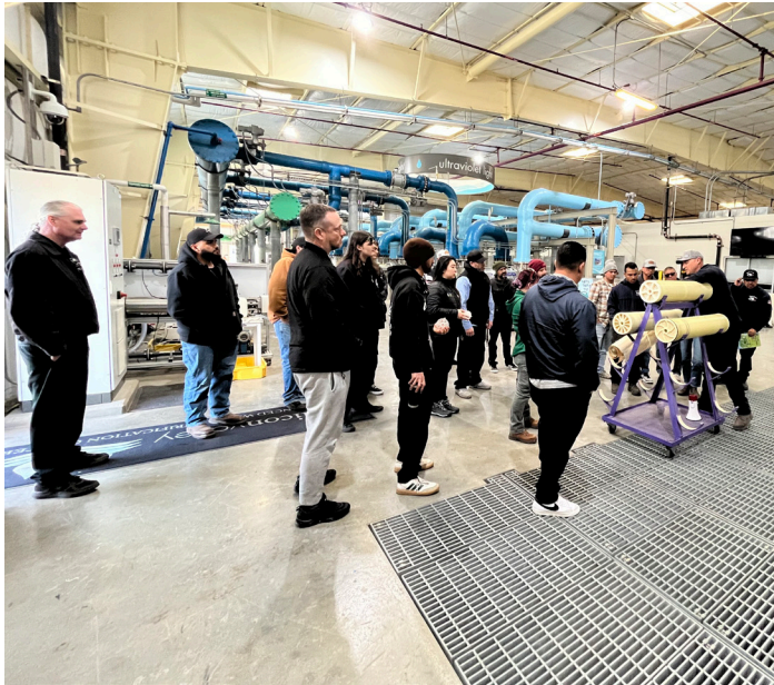
Water industry technicians attend a tour of the Purification Center as part of their cross-connection training with Backflow Prevention Specialists, Inc.
