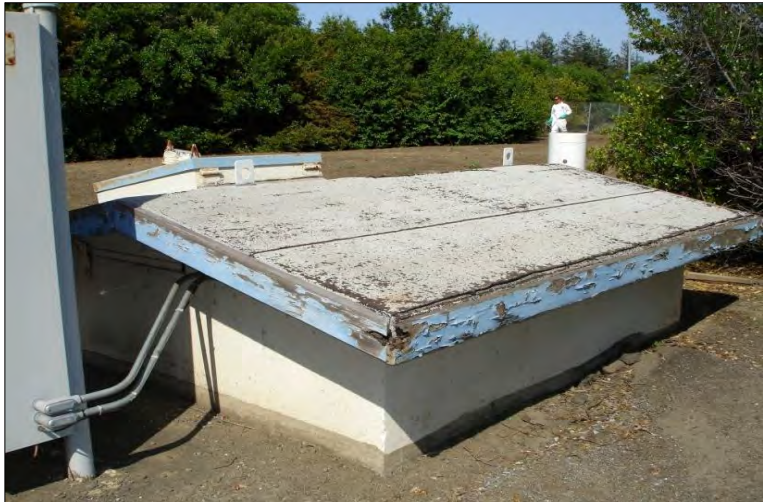
Major repair and replacement of turnout roofs and similar small raw water capital projects will be completed in accordance with the asset management plan.
