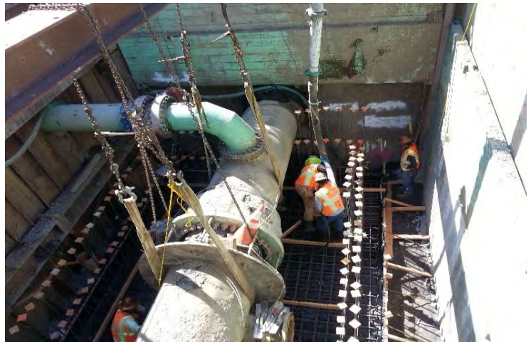
New interties similar to this will be installed in the cities of Santa Clara and Mountain View.
