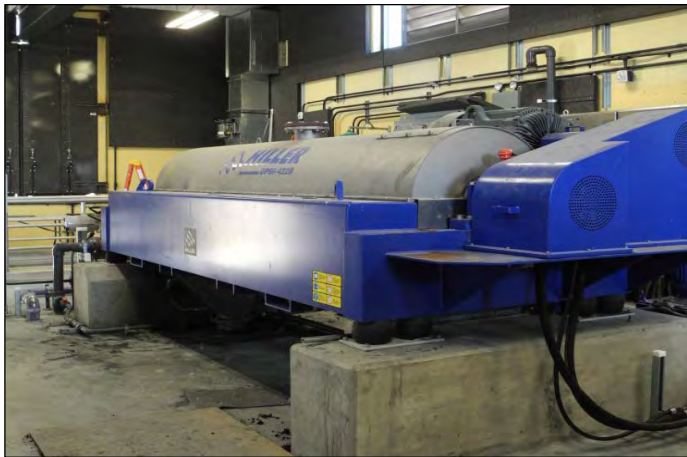
Centrifuge for mechanical dewatering of sludge
