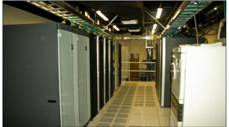
Existing Data Center that houses critical servers supporting Valley Water's normal operations
