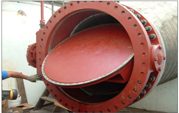
Valve installation in the Piedmont Line Valve Vault; Similar small capital projects will be carried out at treated water transmission facilities according to the asset management plan.
