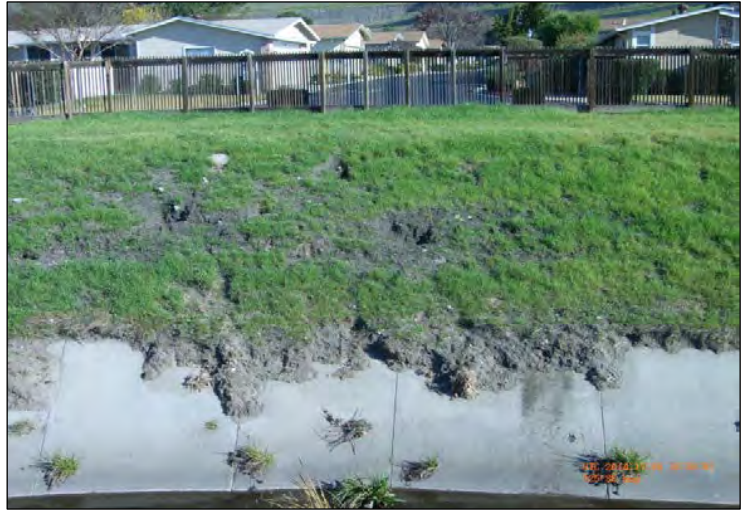
View of damage caused by burrowing animals along Canoas Creek in the Guadalupe Watershed
