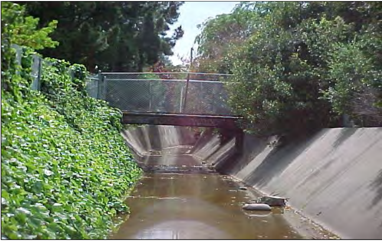
Reach to be modified downstream of 7th Day Adventist foot bridge between Marilyn Drive and North Sunshine Drive
