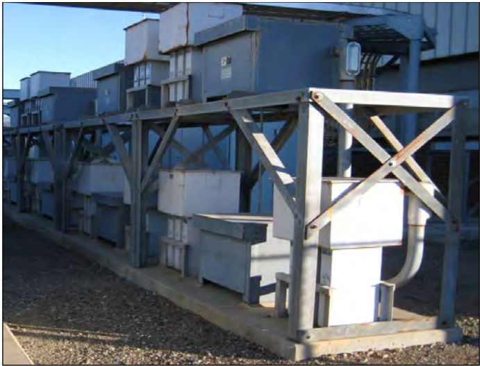
ASD motors at the Coyote Pumping Plant
