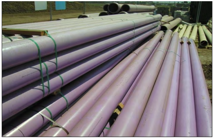
Purple recycled water pipe waiting to be laid during construction of Immediate Term project
