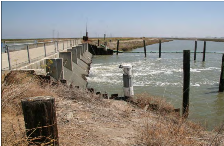
View from the west side of the Palo Alto tide gates facing east
