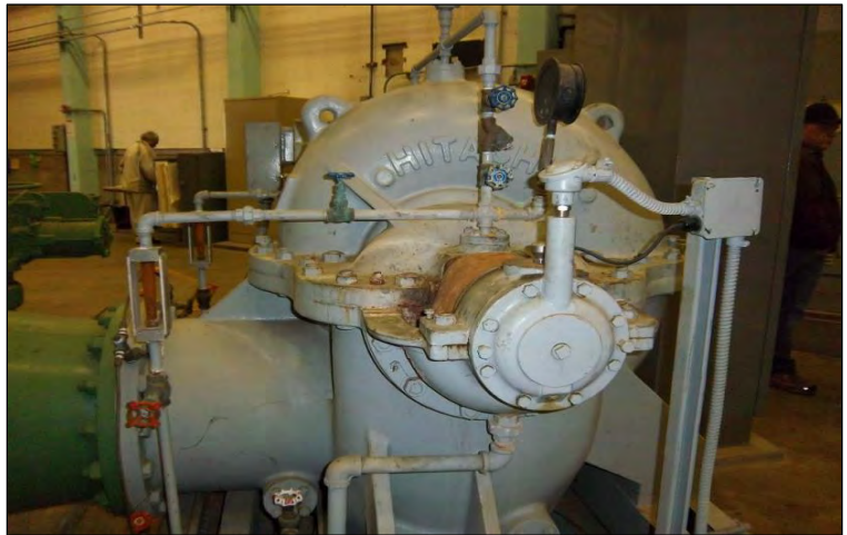
Vasona Pumping Plant pump
