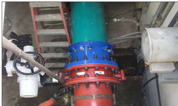
A typical rehabilitated line valve assembly
