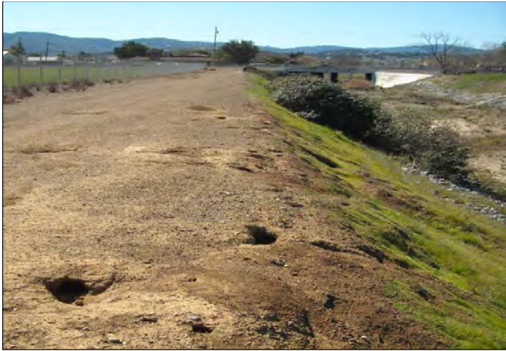
View of damage caused by burrowing animals along West Branch of Llagas Creek in the Uvas/Llagas Watershed
