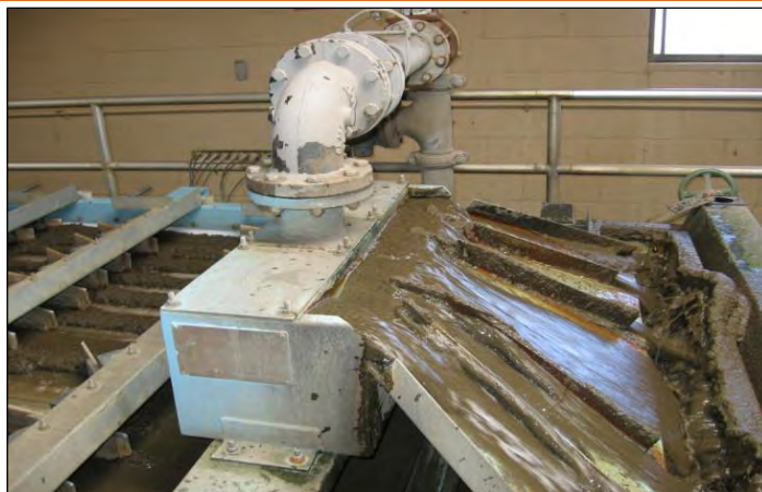
Existing belt press to be replaced with new residuals management facility
