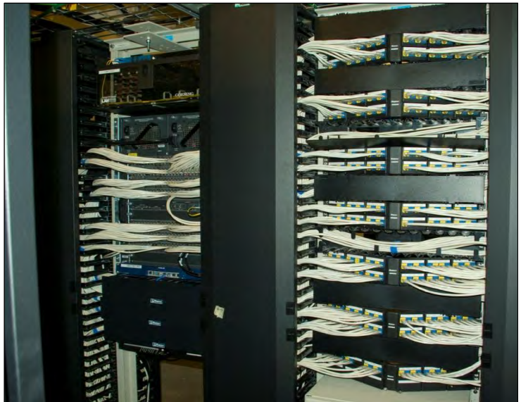
View of network equipment to be modernized at the Water Quality Lab
