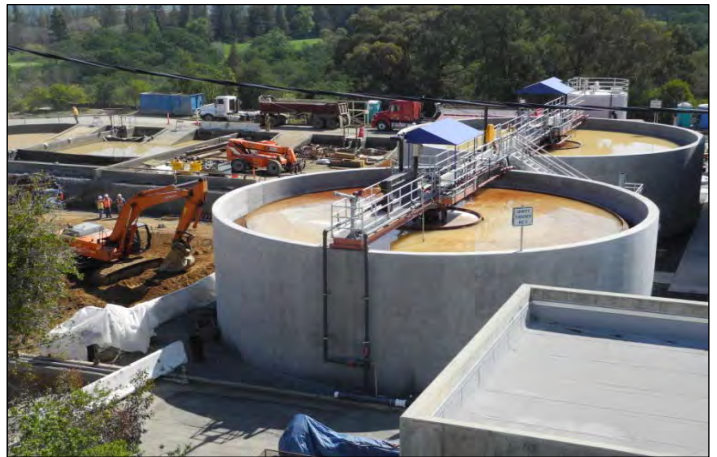
New gravity thickeners and mix tank for sludge thickening and blending
