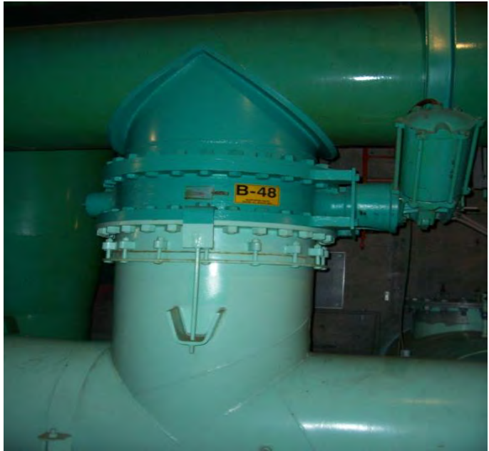
Example of a valve to be replaced or upgraded
