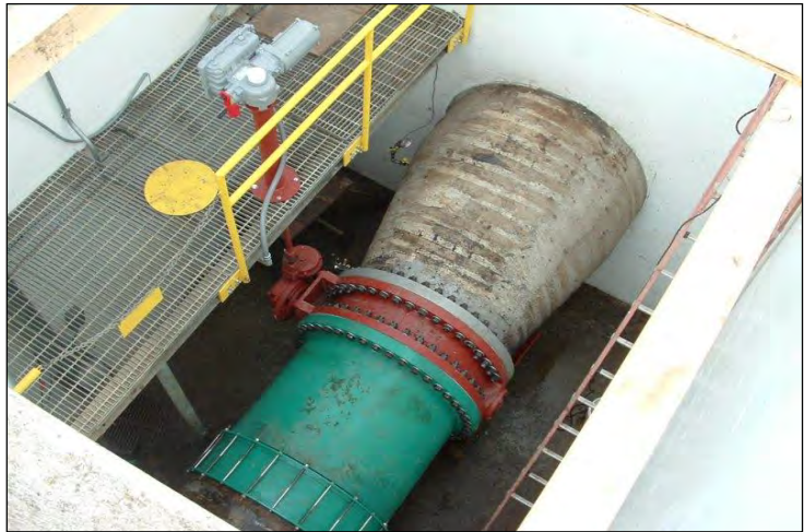
New line valves, actuators, and vaults similar to this will be installed along the East, West, and Snell pipelines
