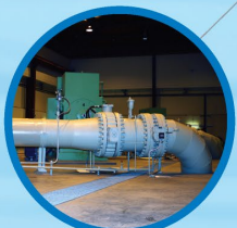
Coyote Pump Plant
