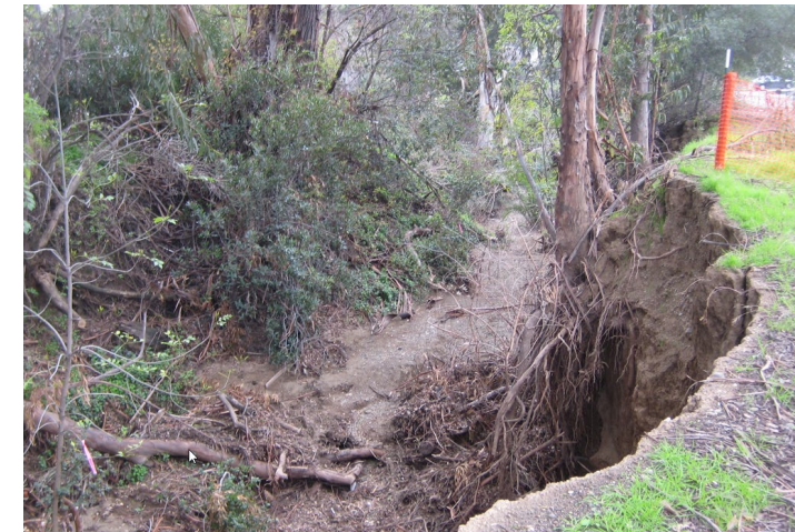
Example of bank erosion – 2016 WARP project
