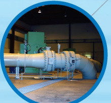
Coyote Pump Plant
