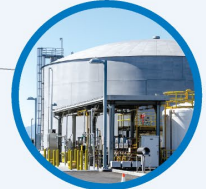
Silicon Valley Advanced Water Purification Center
