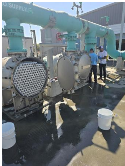
Staff replacing cartridge filter
