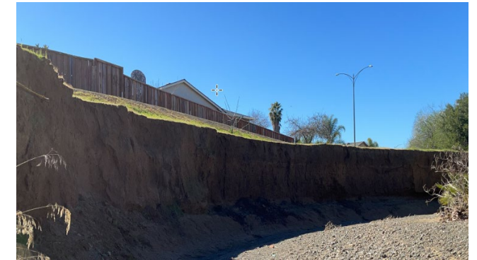
Thompson Creek Erosion – AMP
