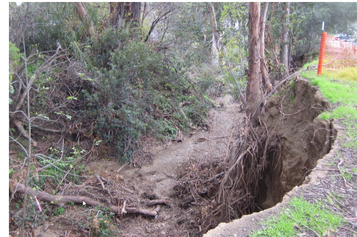
Example of bank erosion – 2016 WARP project
