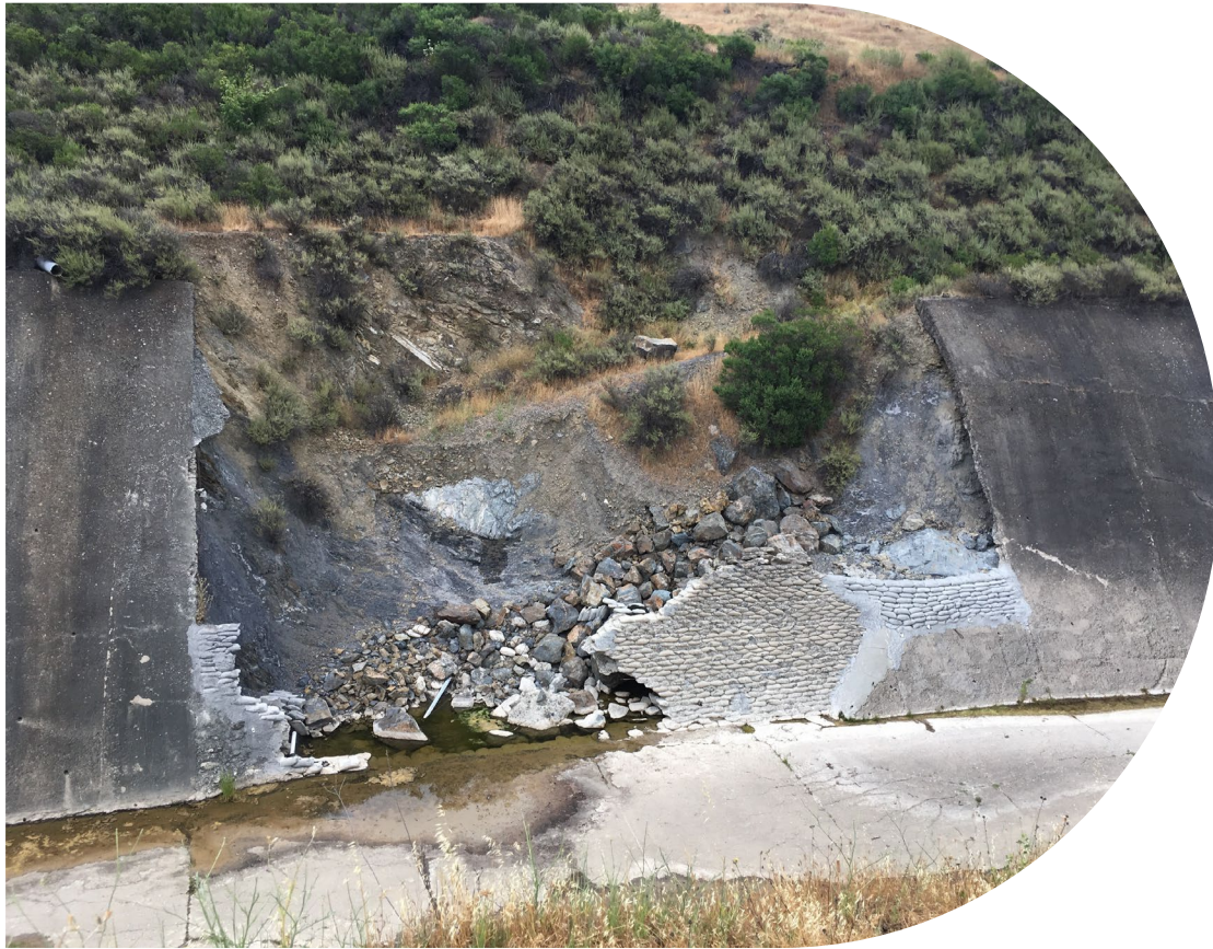
Pictured above: Existing Damaged Spillway of North Fork Dam
