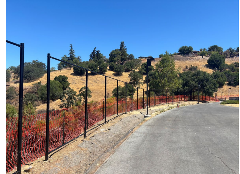
Santa Teresa Water Treatment Plant
