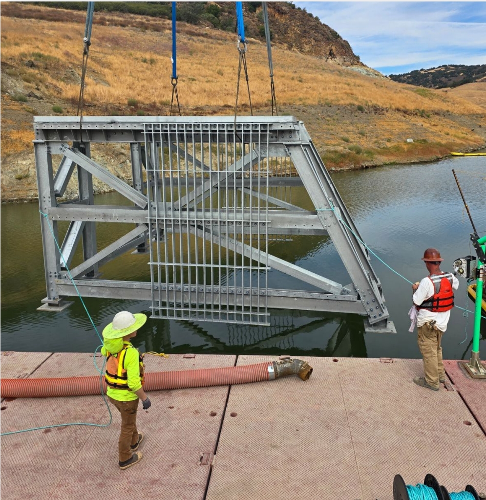
Lake Tap intake trash rack
