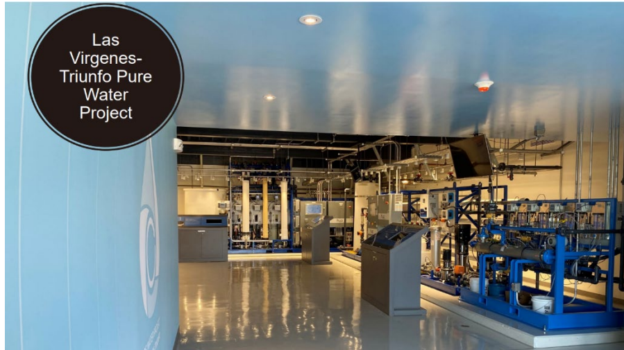
Figure 2: Las Virgenes-Triunfo Pure Water Demonstration Facility Size: 0.14 MGD
