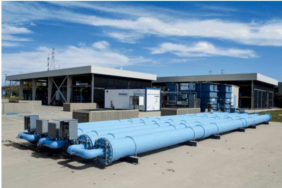
Figure 6: City of San Diego Pure Water Program – Demonstration Pure Water Facility Size: 1.0 MGD
