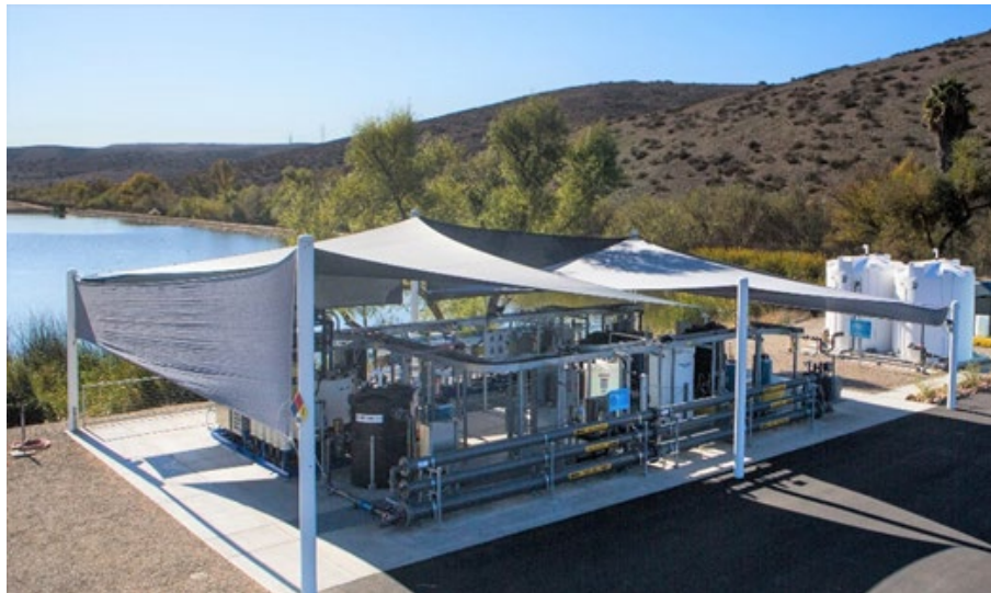
Figure 3: East County Advanced Water Purification Program (Padre Dam) Size: 0.1 MGD
