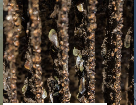
Skinner Fish Facility Louvers - 2025 Courtesy of DWR
