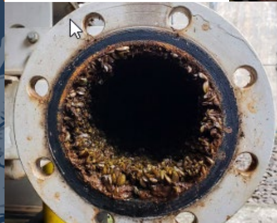
Golden Mussels colonizing a water pipe at a hydroelectric plant in Brazil (Mountinho, 2021).
