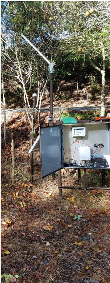
New stream gauge sensor.
